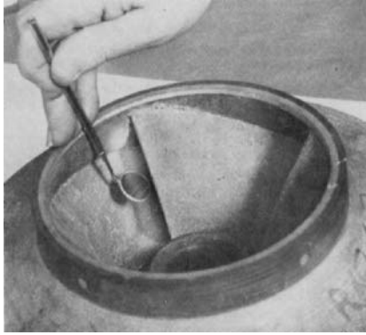
FIGURE 1 Examining the pressure side of the inlet vanes for suction recirculation damage
